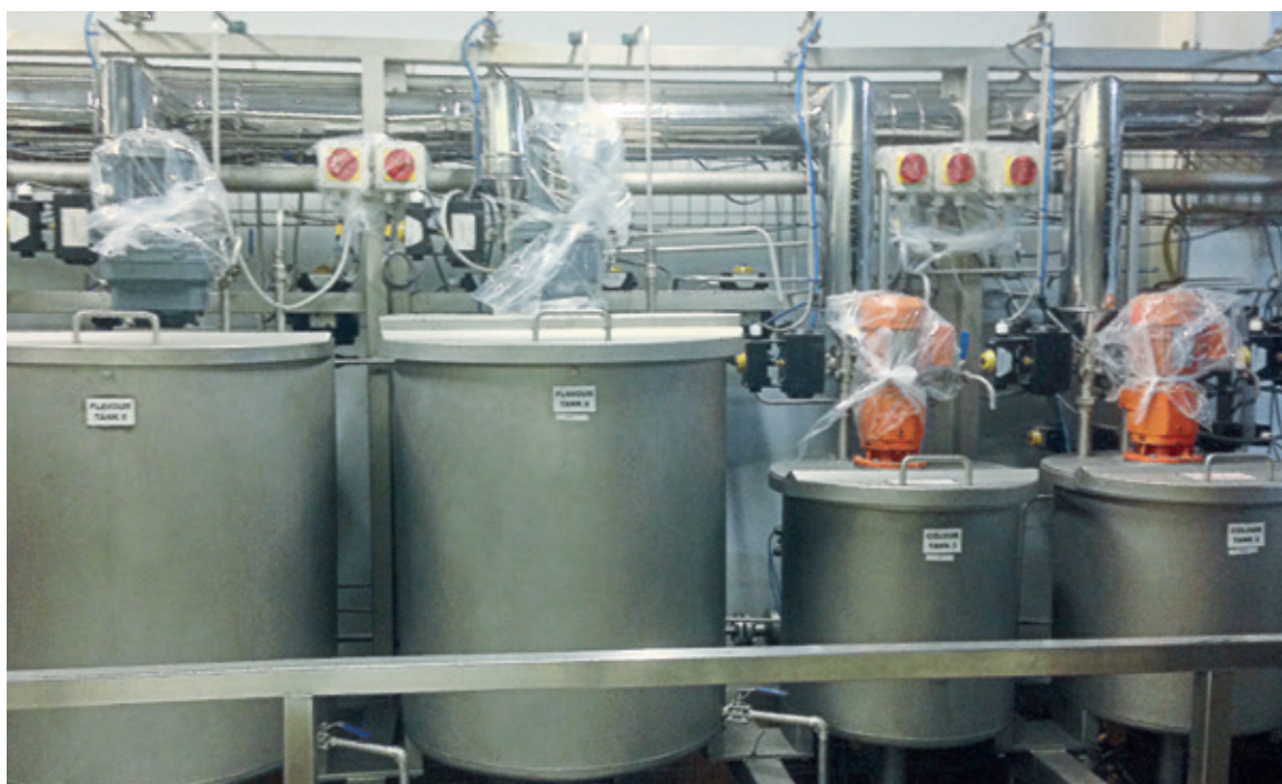
Holding tank for multiple ingredients.
