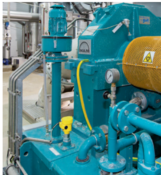
Level measurement in the lubricating oil storage tank of the vacuum pump.
