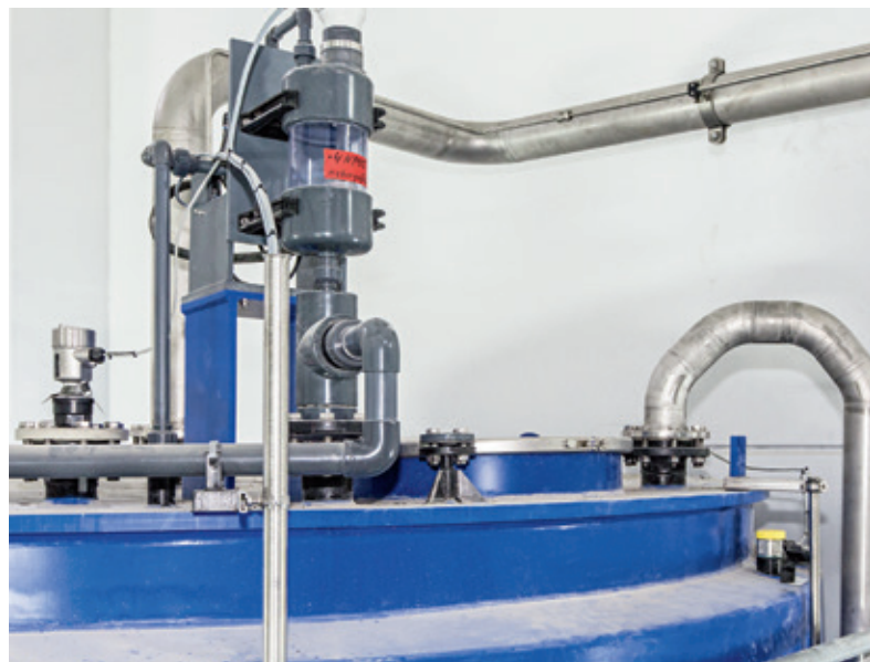
Level measurement and leak detection in the storage tank for wet strength agent.
