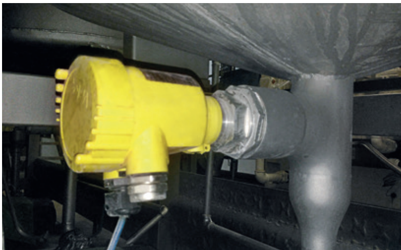
Level measurement in holding tank with VEGABAR 82.
