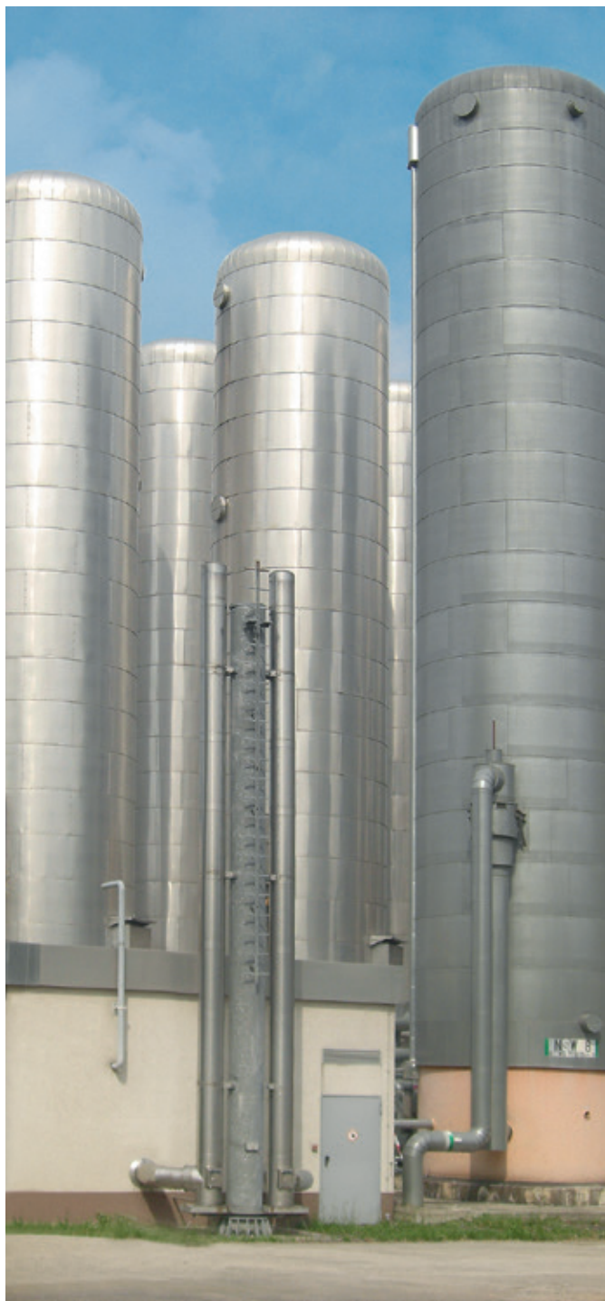
The equalization tanks ensure optimal pressure in Leipzig's district heating network.
